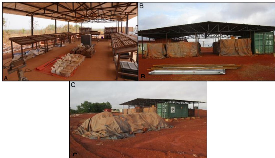
Figure 12.1 – A) Core logging facility; B) Core storage hanger; C) Protected temporary storage for rejects
