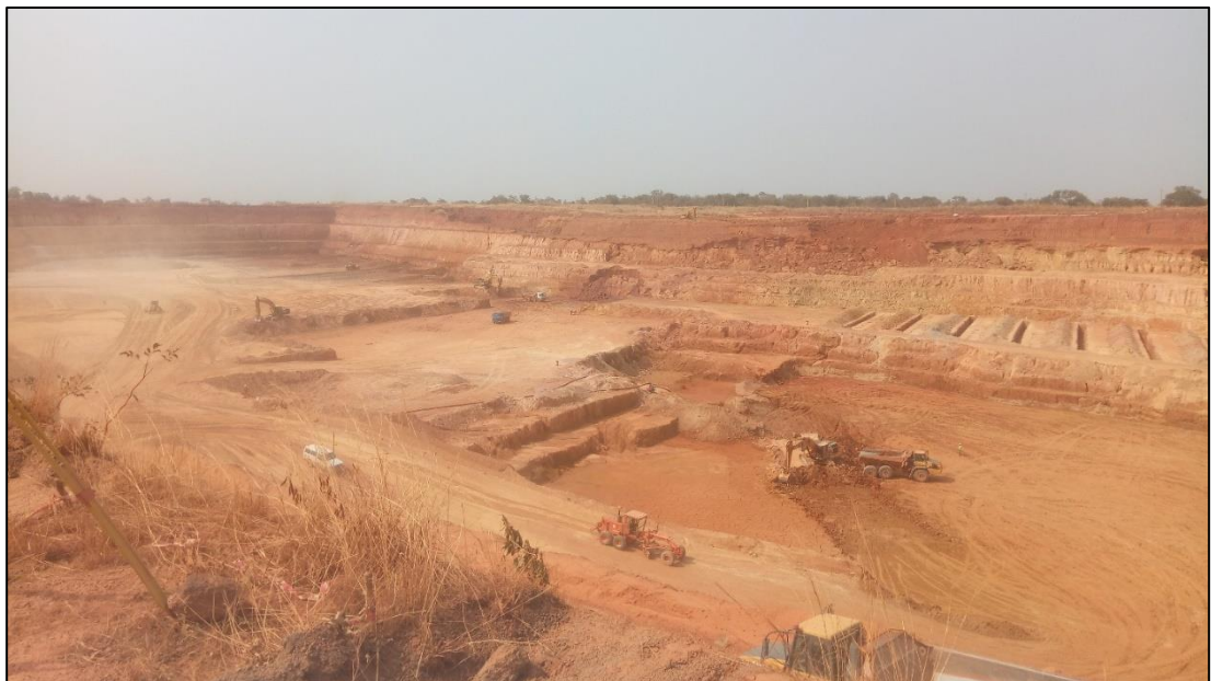
Figure 5.6 – Photo of the Nampala open pit in production, looking west (photo taken during April 2017 site visit)
